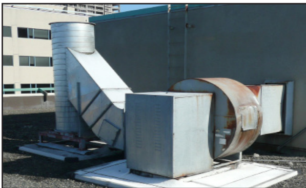
Original exhaust fan and duct work.
