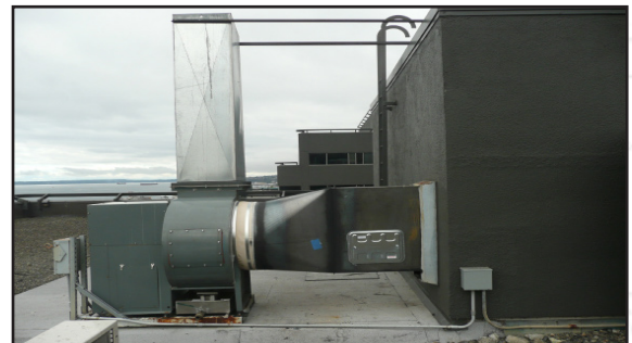
New exhaust fan and duct work.
