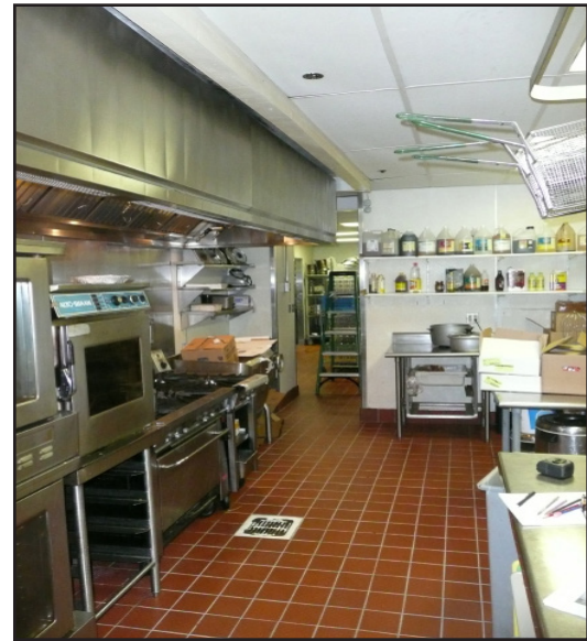
One of the 3 large cooklines supported by the exhaust system upgrade.
