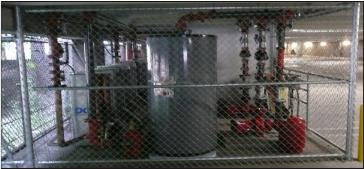
The new central plant. Key components include 97% efficient gas boilers, redundant pumps and dry coolers.
